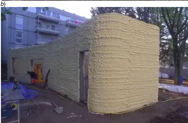
Fig. 6. House made according to the project of scientists from the University of Nantes in 3D printing technology: a) finished building, b) skeleton of walls [22]
